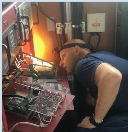
EM1 William Gore inspects a battery charger.
